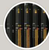
TRACKSIDE AUTOMATIC TRAIN CONTROL SYSTEM
