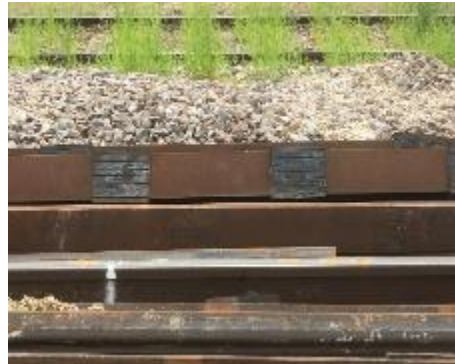
Figure 17 : used pads stuck underneath the rail
