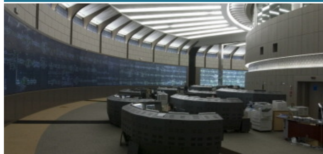
Centralized Train Traffic Control Center
