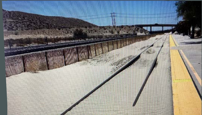
Sand ingress at Palm Springs Station, California ©AMTRAK
