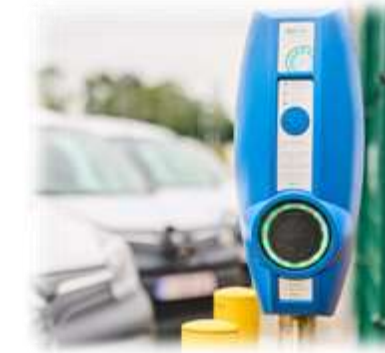
Electric feed for EV charging
