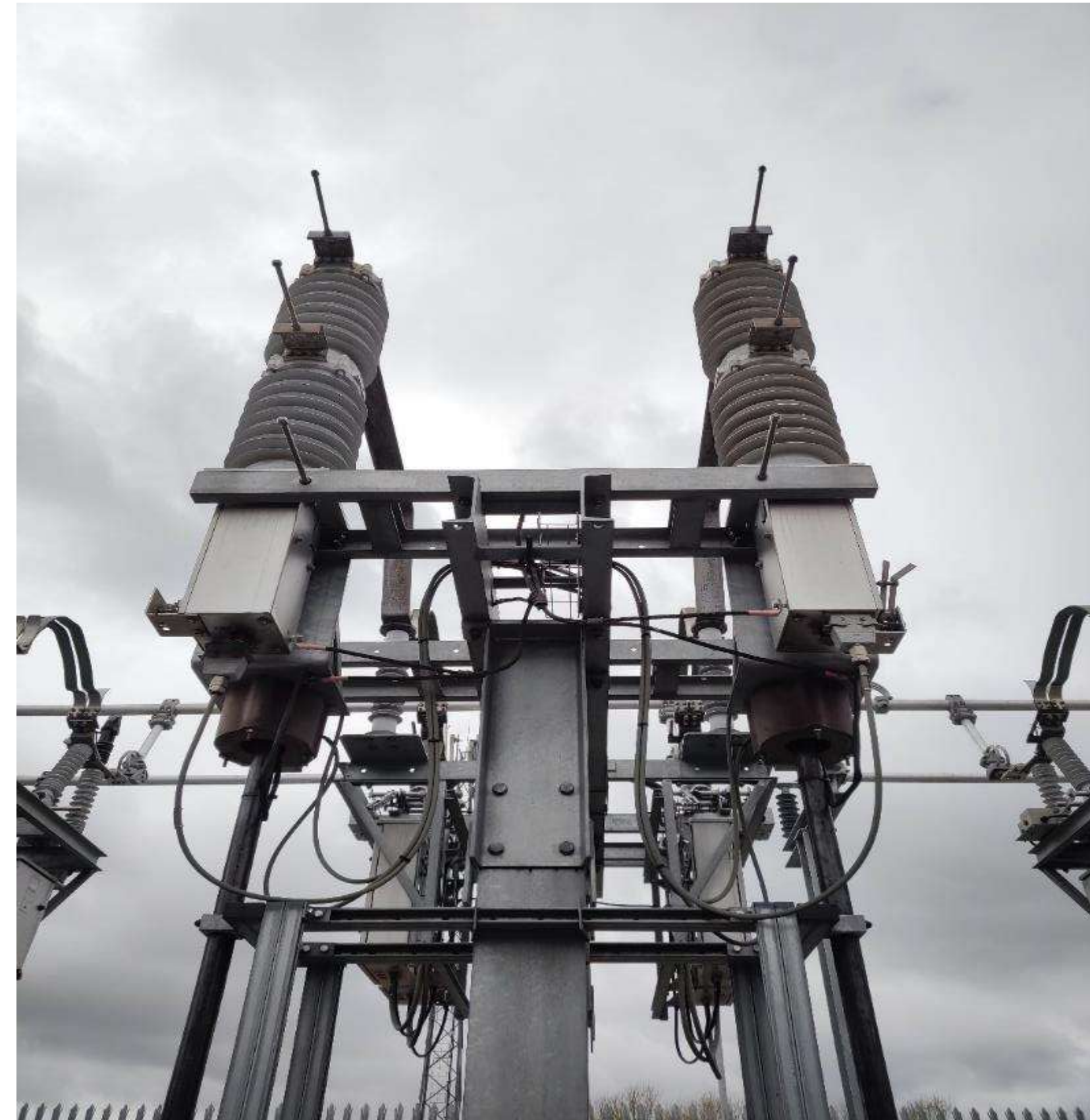
Empty bay with two 25 kV circuit breakers and the +25 kV & -25 kV busbar in the background.
