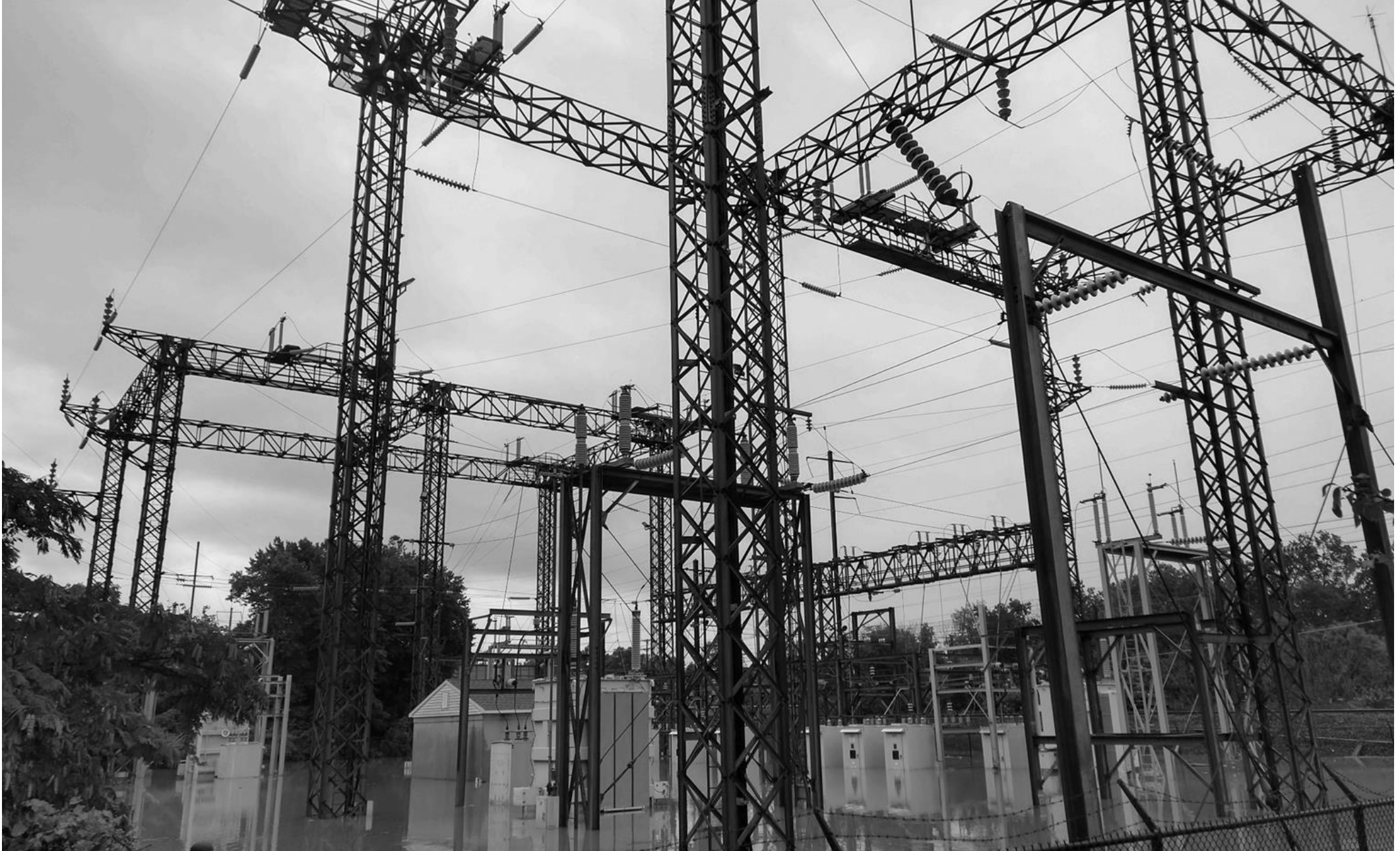
-Landover Substation, September 1, 2020
